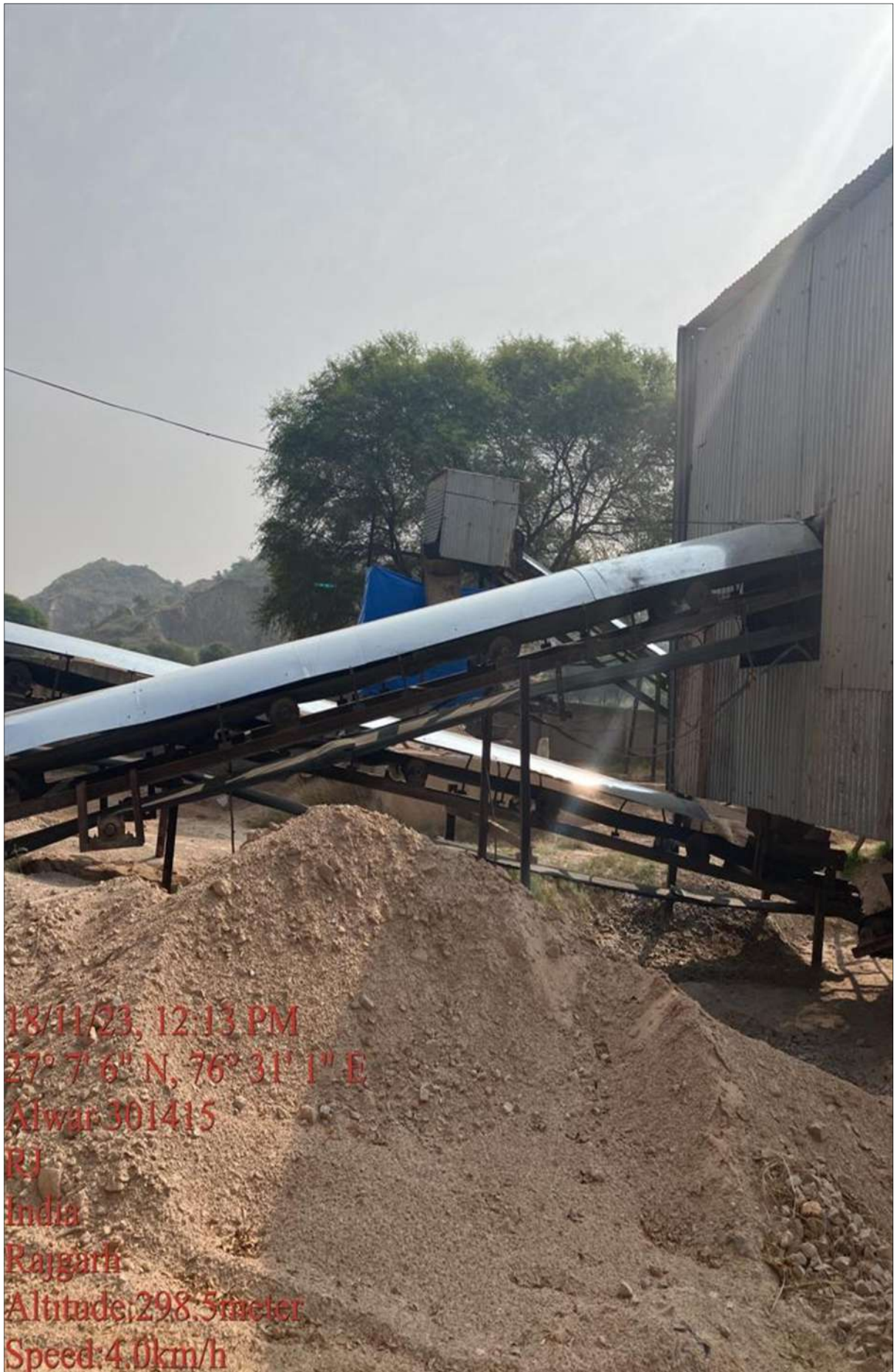
Fig 03: Covered material transfer conveyors.
