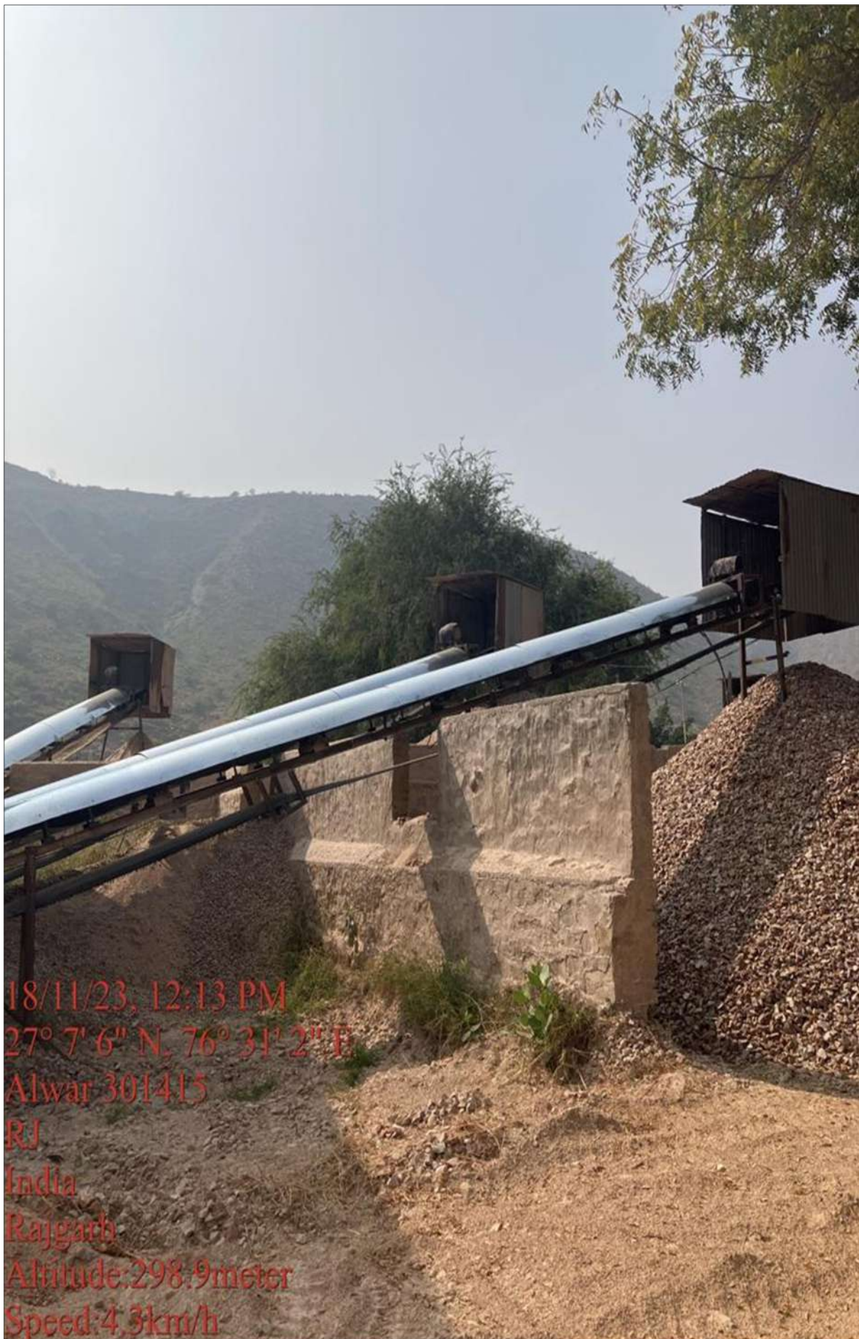
Fig 04: Covered delivery conveyors.
