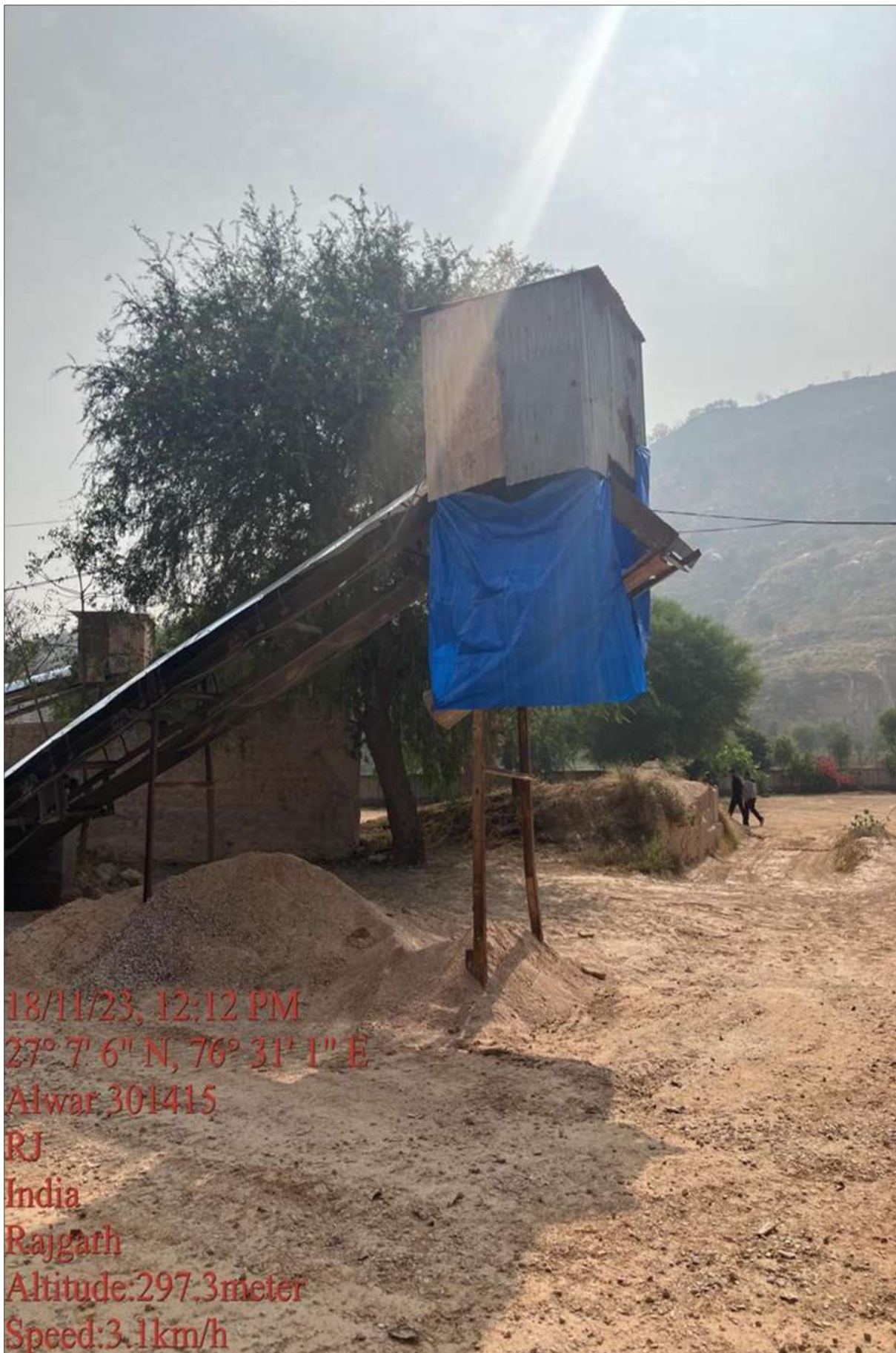
Fig 05: Arrangements at the falling point of conveyor to reduce the dropping height of material (for size less than 05 mm).
